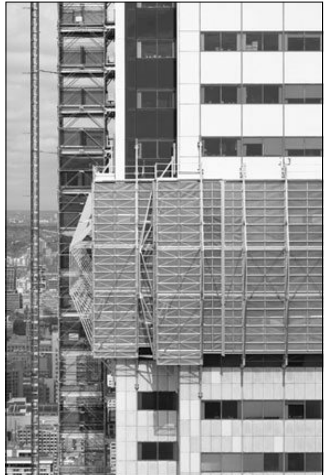
First Canadian Place. Note the discoloured marble below the three-tier scaffolding, and the newly installed white glass above.
